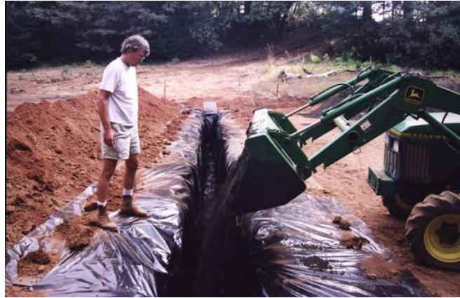
Figure 2.8: The first trench was lined with plastic and filled with sand and water. The second trench was not lined with plastic. field-fill_1 [NR]
